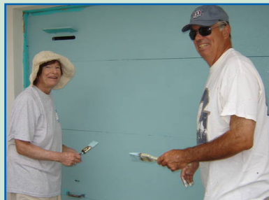
Project coordinator – Cathy Maloy and husband Paul put finishing touches on the garage for Rebuilding Together.
